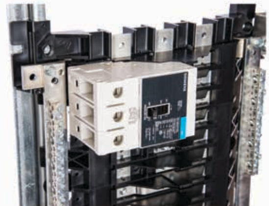
Example of Back-fed xGB Main breaker installed
