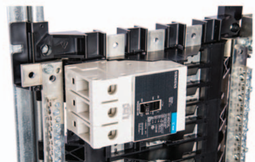
Example of Back-fed xGB Main breaker installed
